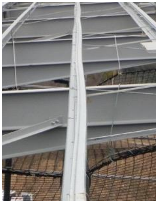
Excessive purlin rotation before any load applied
